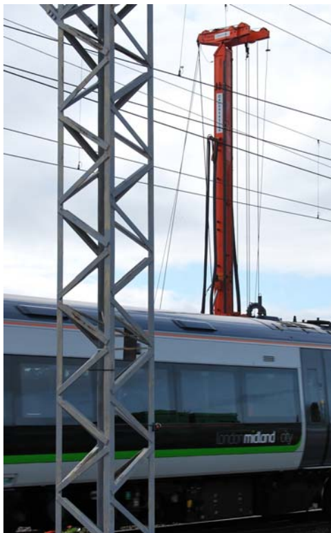
Pictured above: A piling rig works close to the busy West Coast mainline whilst the Leica equipment and GeoMoS software monitor the track for movement.
