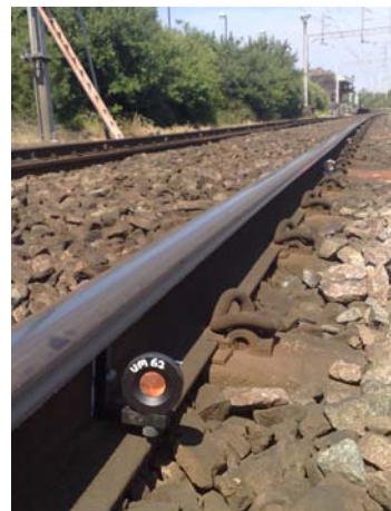
Pictured above: One of the 300 mini prisms fixed to the rails to monitor the track.
